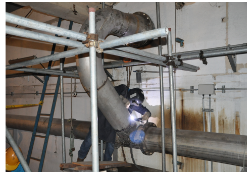
STAINLESS STEEL PIPING
