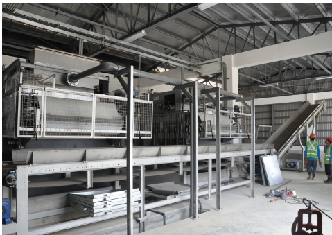
SLUDGE BELT PRESS
